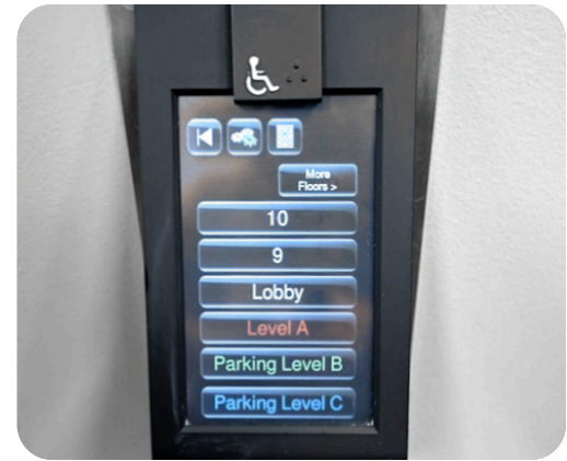
Destination elevator touchscreen
